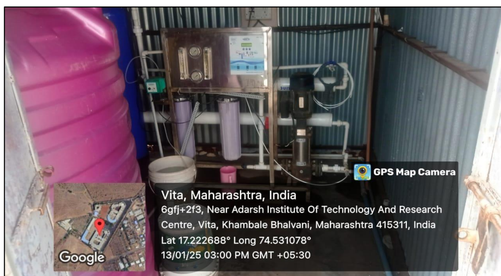
Figure: RO plant at institute
