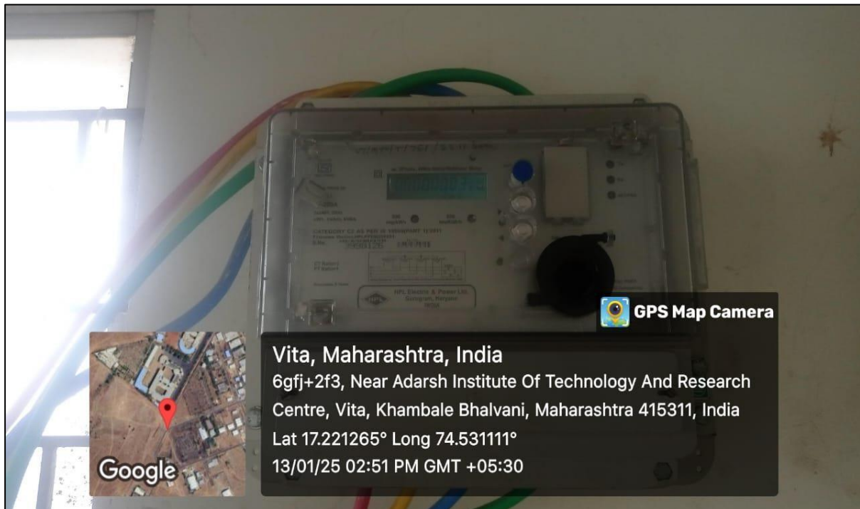
Figure Energy Meter
